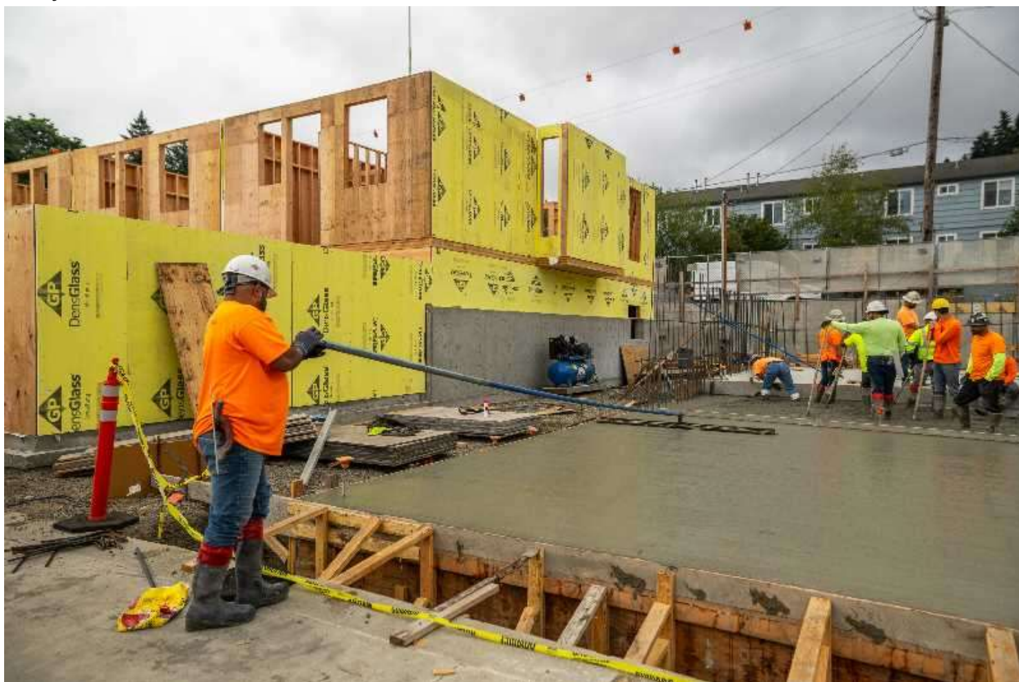
COURTESY PHOTO: NOEL JOHNSON - Workers lay the foundation at developer Noel Johnson's cross-laminated timber Wilson Forest Park Townhomes in Northwest Portland. Johnson said the permitting has taken three and a half years, for a building that takes just eight months to erect.
