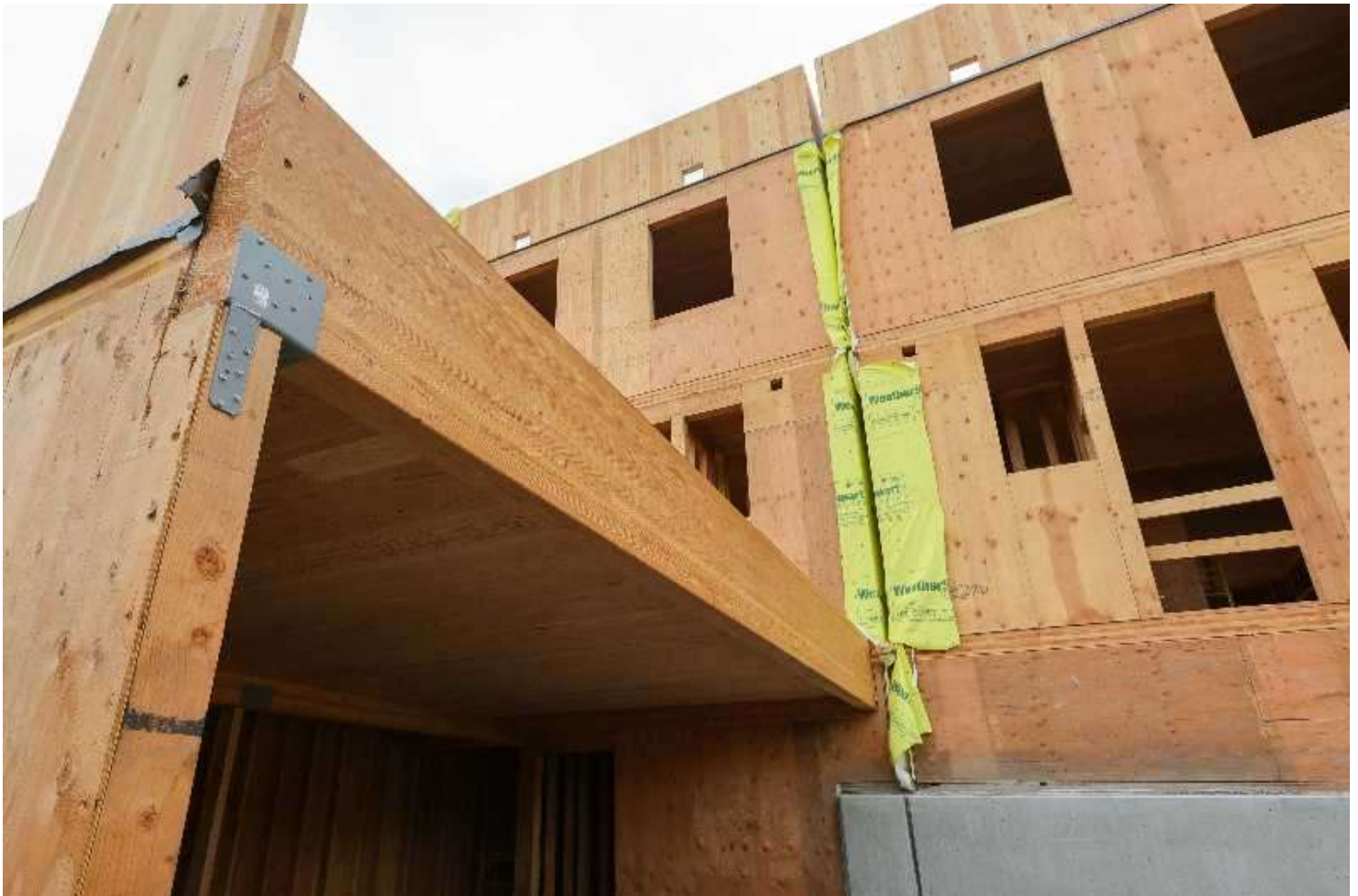
PMG PHOTO: JONATHAN VILLAGOMEZ - A garage space at the Wilson Forest Park Townhomes in Northwest Portland, with a large deck above it. The cross-laminated timber townhomes are deliberately kept four and a half inches apart (at the yellow fireproofing film) so that they can't be considered condominiums.
